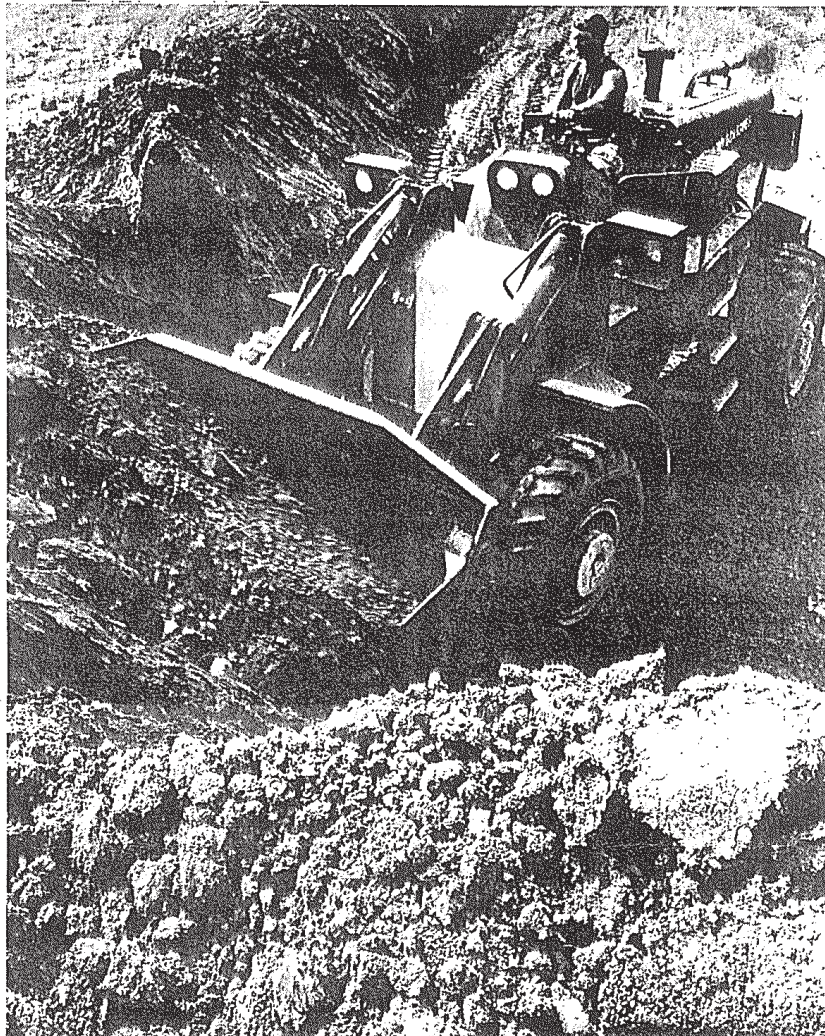
DIGGING IN -- A member of the 4th Engineers makes full use of his machinery while forming Camp Radcliff into a Division nerve center.
